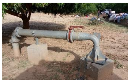
Borehole and valve
