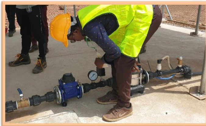
Photo 6: Studying the solar irrigation pump is vital
