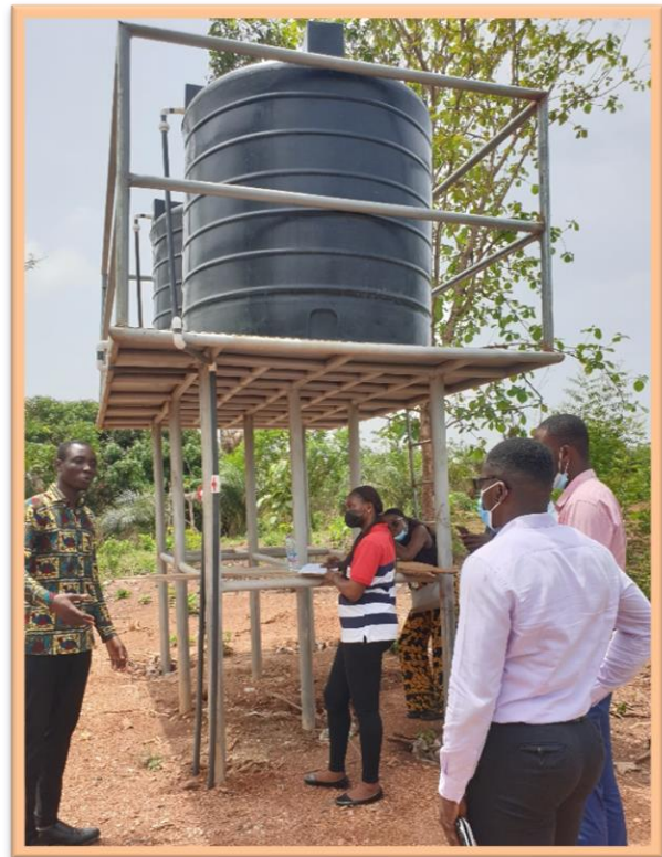
Photo 7: A water reservoir tank on an elevated platform
