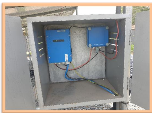
Photo 8: Control devices of a solar-powered irrigation system in protective box that can be locked
